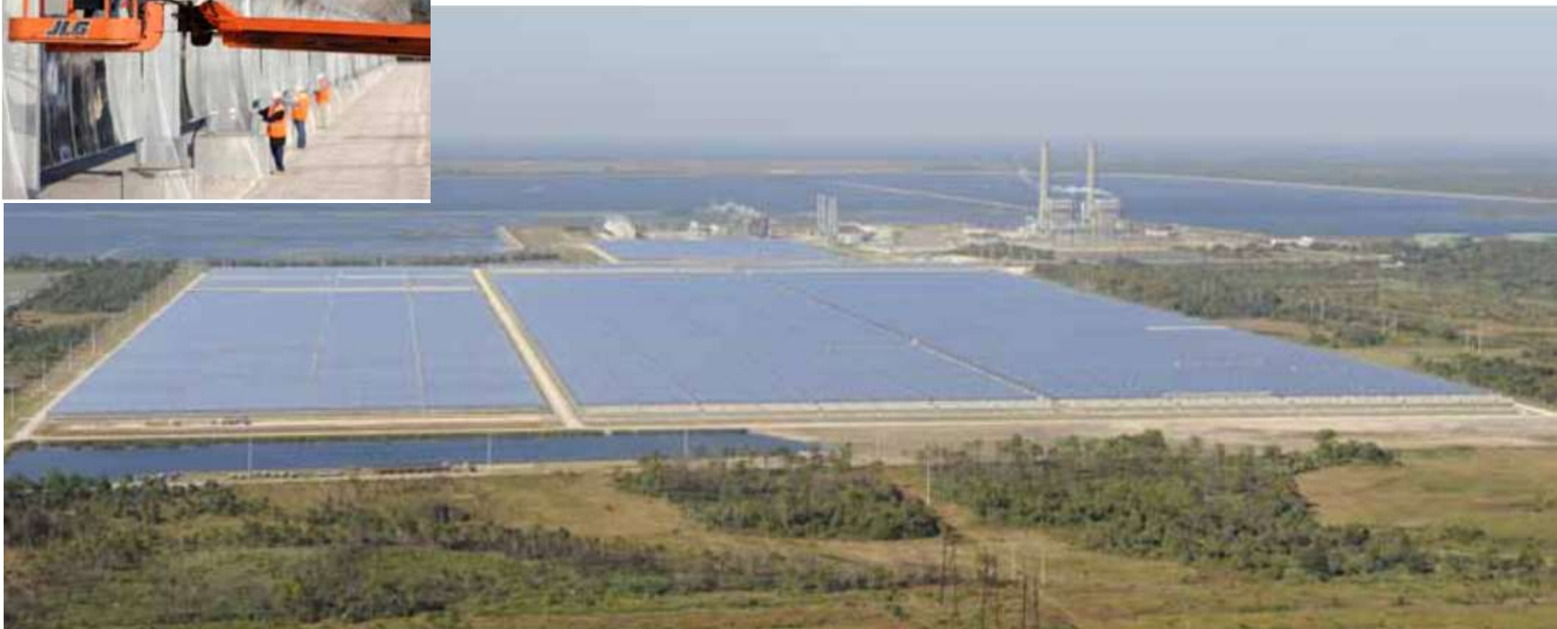
75-MW Martin Solar Plant near Indiantown, Florida
